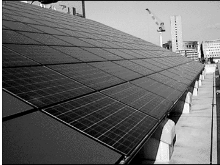
fig.7 Yono Institute, The Dowa Fire & Marine Insurance (20kW)
