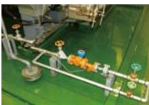
A fuel oil flow meter
