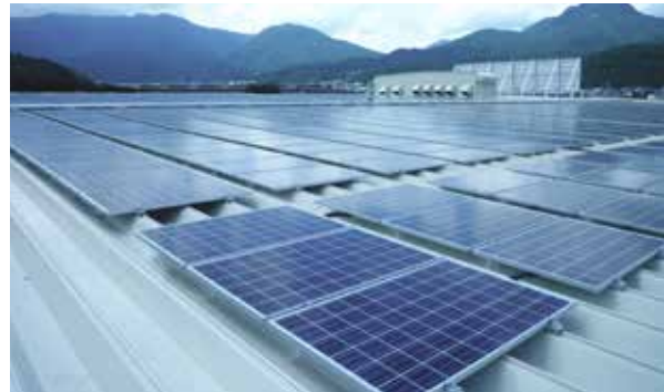
Solar panels at Logistics Center
