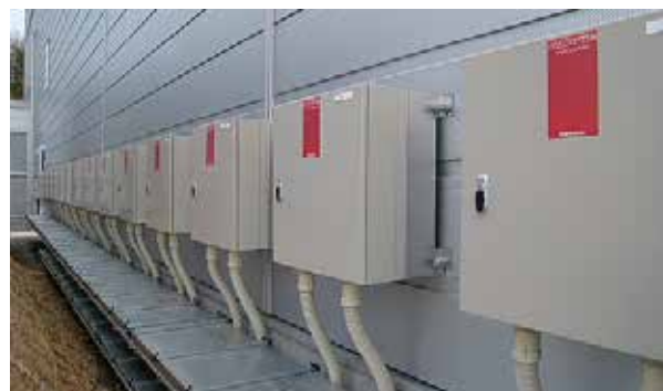
PV Inverters at Fujiyama Works
