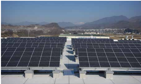
Solar panels at Kangawa Works
